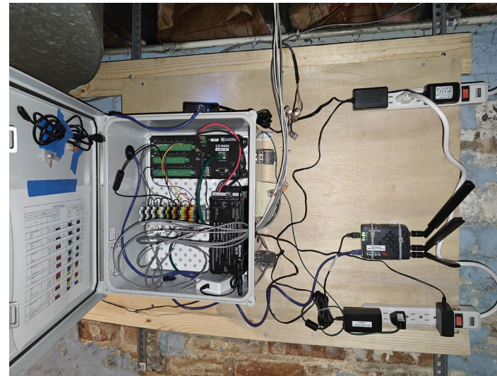
Data logger and communications board
