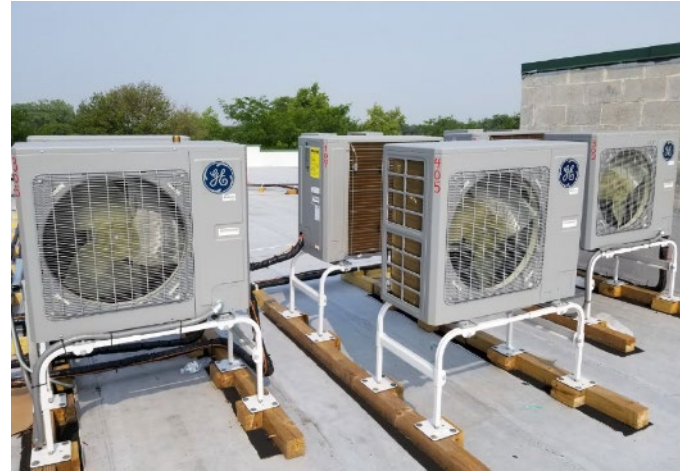
Cold climate air source heat pumps installed for a multifamily Whole Home Electric project. Credit: Elevate
