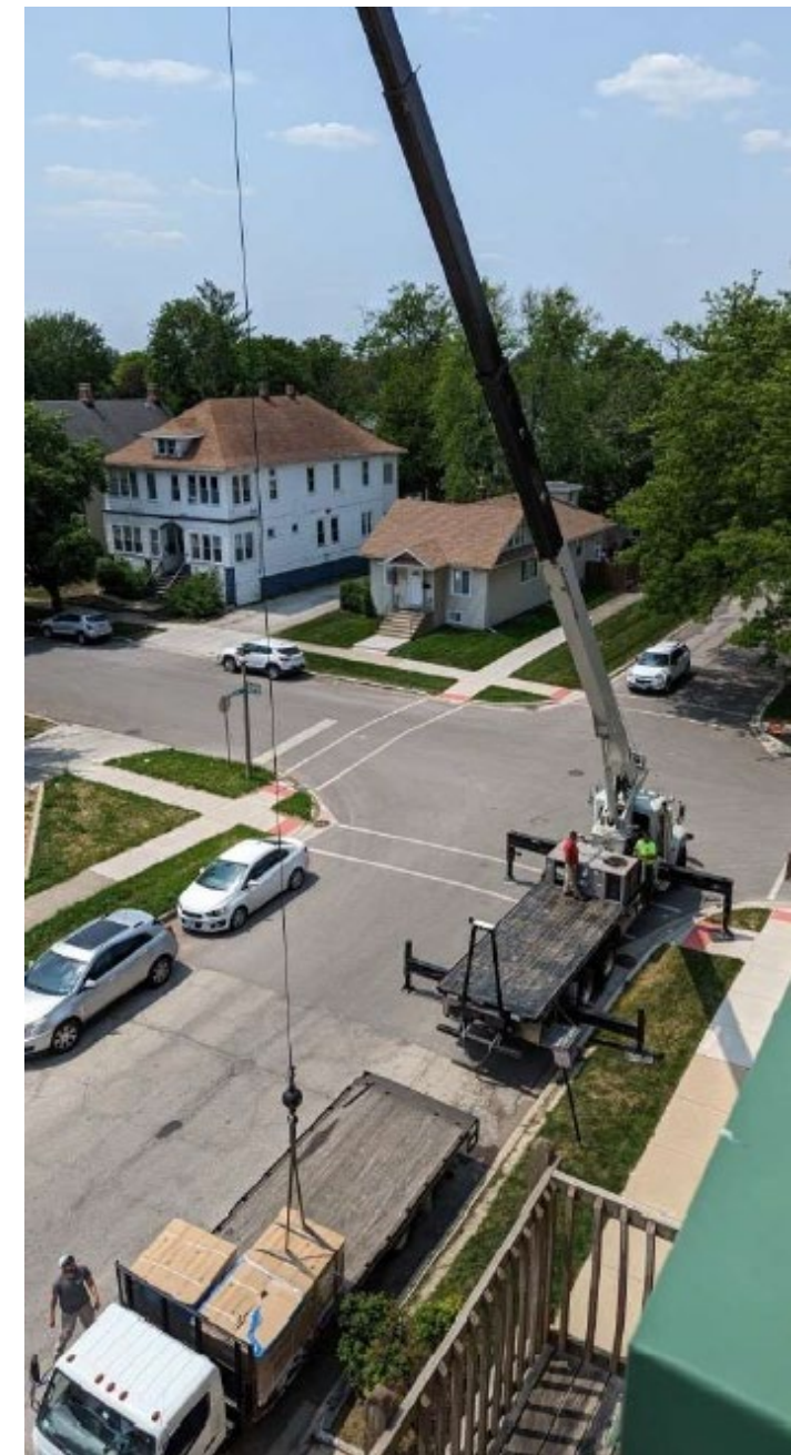
Heat pump equipment is lifted onto the roof of a multifamily building in Maywood, IL. Credit: Elevate
