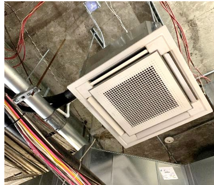
VHE DOAS HVAC installation at Oak Park Temple, Oak Park, IL.
